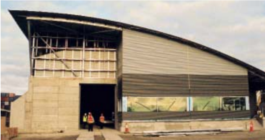
The container x-ray scanning hall stands 12.5m high and is 43m deep: in Melbourne the facilities have been built on silt so 25m pylons were sunk into the ground to stabilise the structure.
